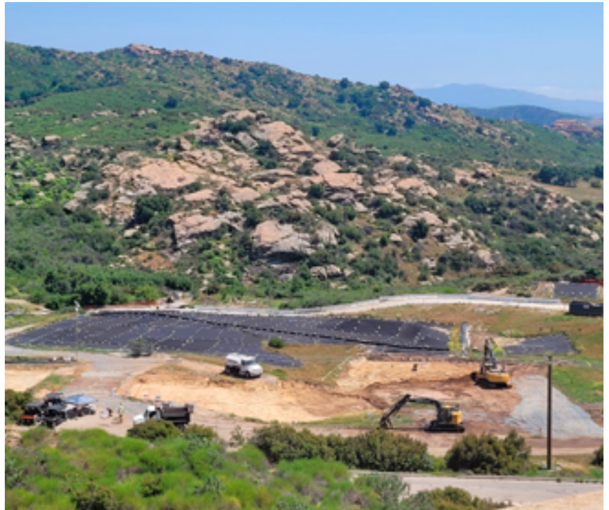
The DTSC-ordered cleanup of the Area I Burn Pit will remove an additional 10,000 cubic yards of soil
