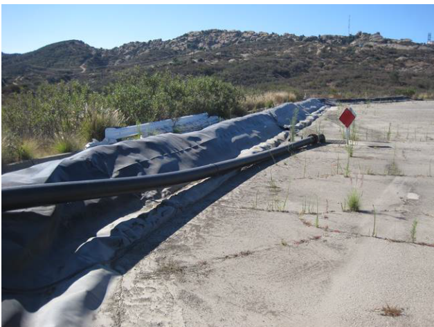
2011: Helipad Berms and Pumps
