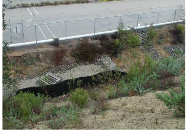
2012: B-1 Sedimentation Basin and Media Filter
