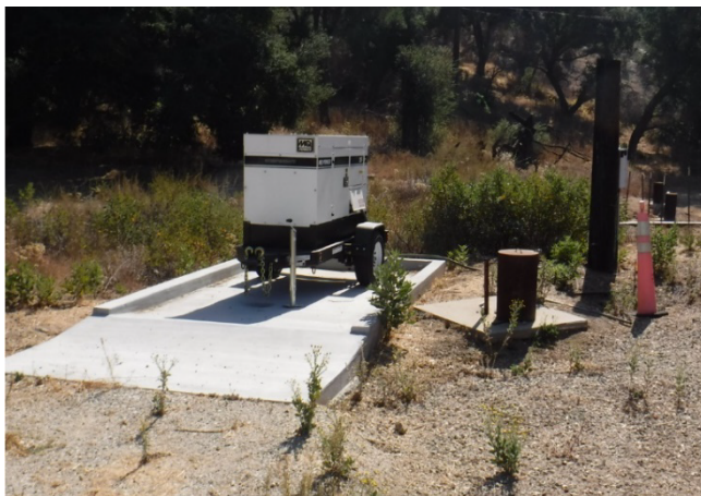
2020: Outfall 009 ELV and Biofilter Cistern Generators Added
