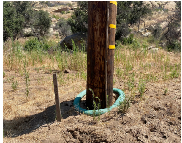
2020: Southern Buffer Zone Utility Pole BMPs
