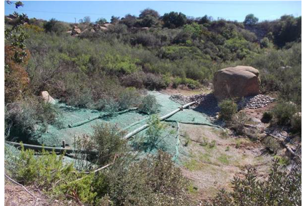
2012: CM-9 Additional Improvements (Perforated Pipe, Extended Sedimentation Area and Rip Rap Berm)
